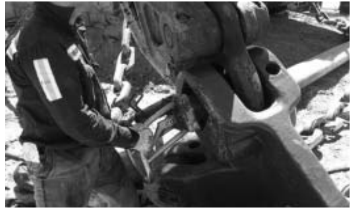
Apprentice boiler maker Michael Ede has designed a pin handler to reduce the risks of performing maintenance on the dragline.
